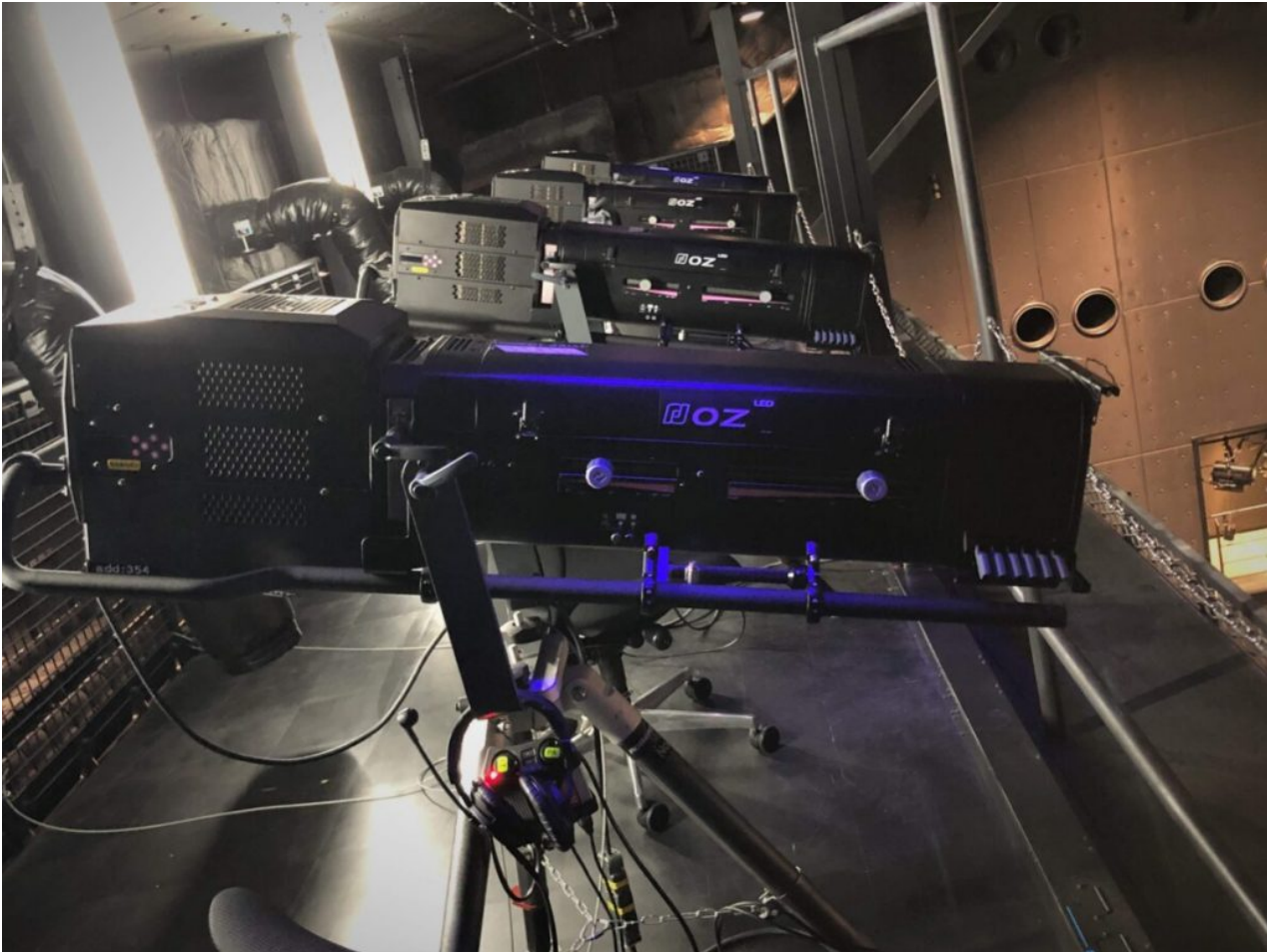
RJ Oz followspots installed FOH at Zepp Haneda
