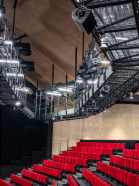
L-Acoustics X8 are mounted on the truss for delay in The Galabru theatre.
