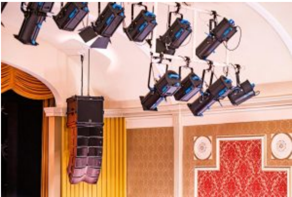
Close up of Schouwburg Ogertop's L-Acoustics Kiva II main system.
