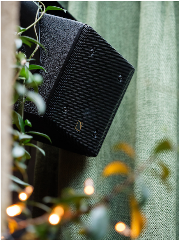
The Roof Gardens’ new L-Acoustics
