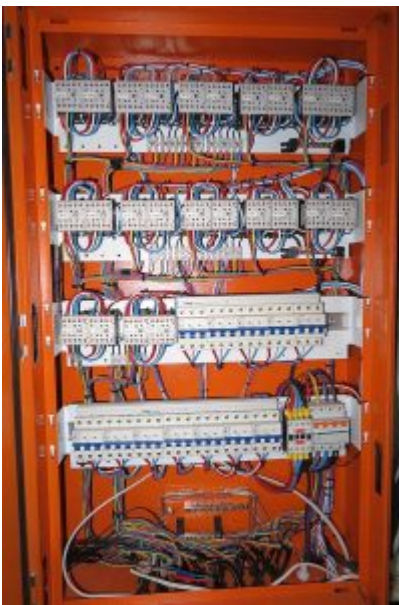
Motor control board for Fly Bars
